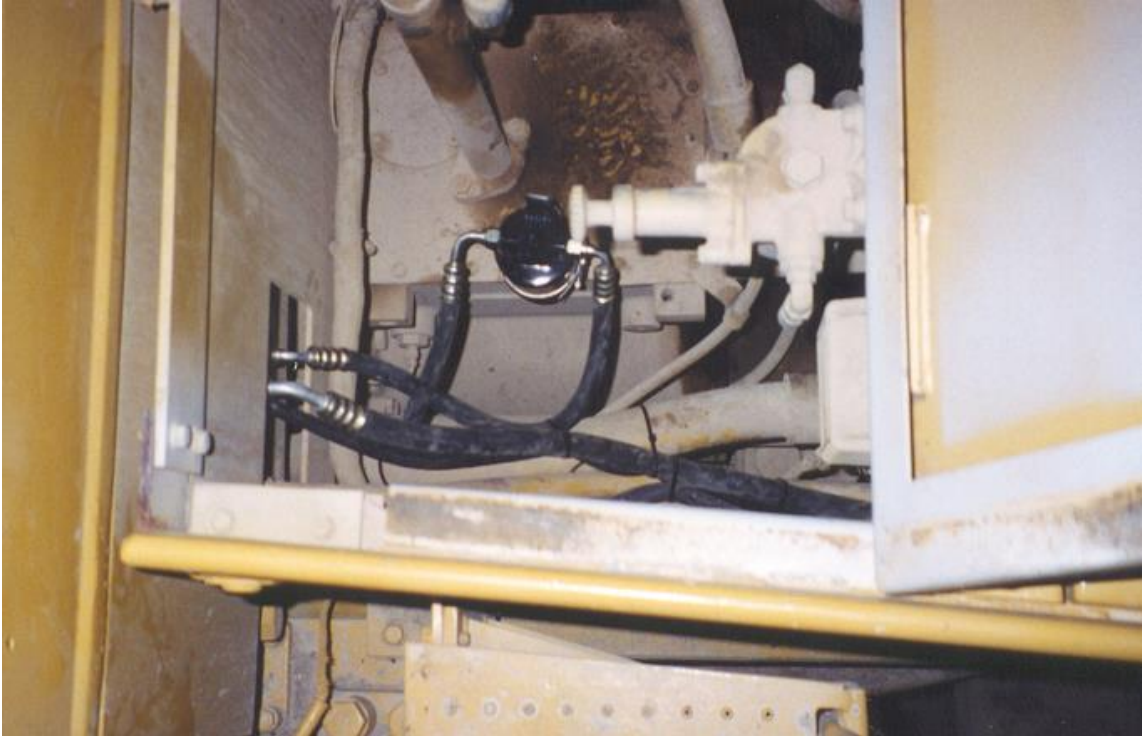
Drier in place with hoses.
