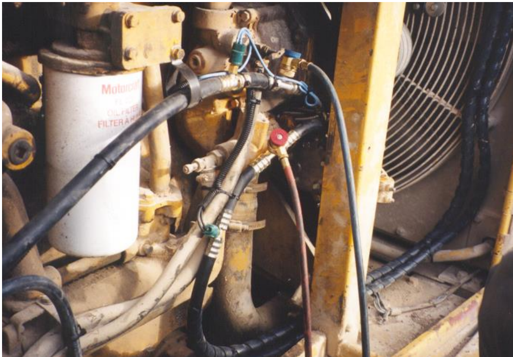
Hoses at compressor and bottom of radiator shroud.
