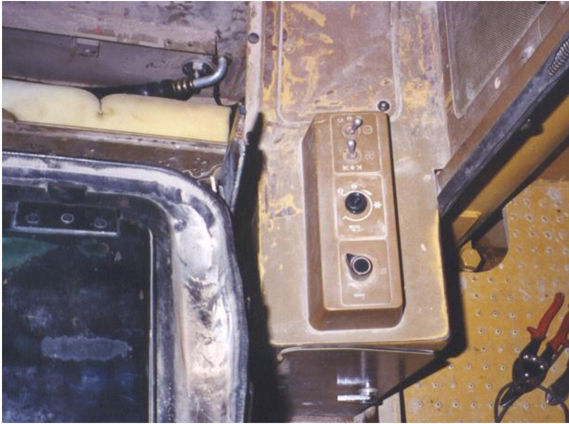
Thermostat in position.
